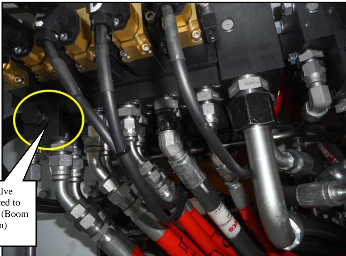
Figure 2: Location of HAWE 5-section valve bank, with relief valve block highlighted
